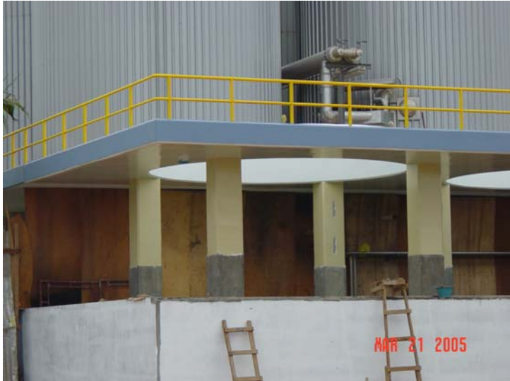
CBL-Tank Room Extension Project Robos Angkagne, Kien Svay, Kandal Province Owner: Cambodia Brewery Limited
